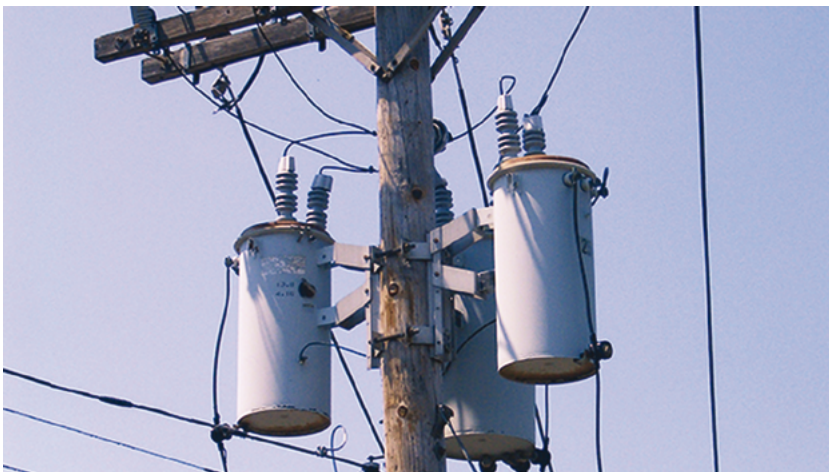
Local power distribution comes from a final stepdown transformer that takes one phase of the grid power and creates the split-phase 120/240 VAC commonly in use today.
