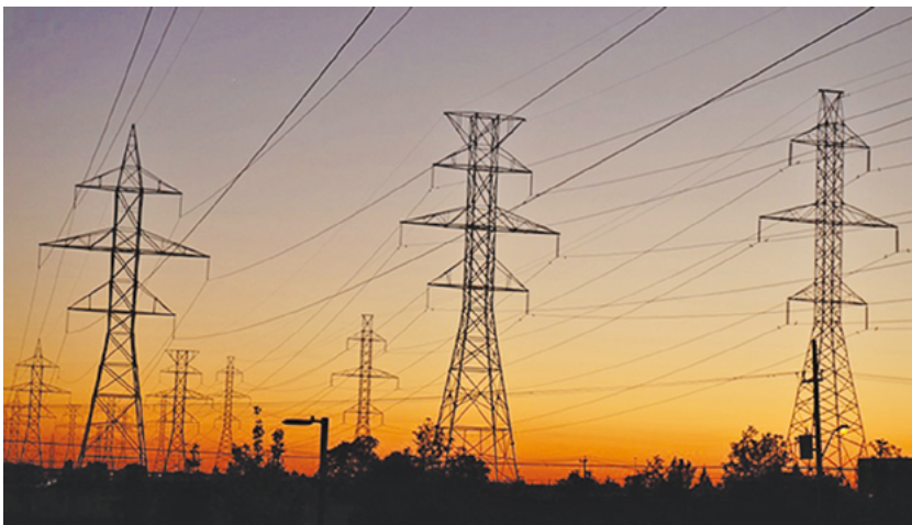
High-voltage power transmission on the grid is generally done as a three-phase power system until it reaches the local distribution point.
